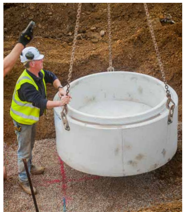
Top Tip - Clean inlets and outlet of any debris
